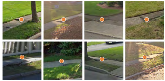
Figure 12: Project Sidewalk Oradell surface problems labels showing height differences on sidewalks and uplifts caused by tree roots.
