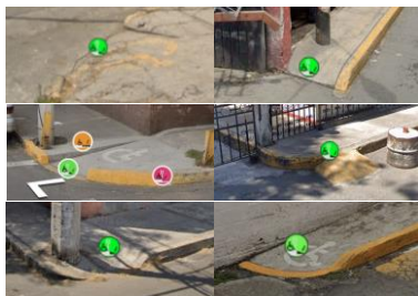
Fig. 5: Example curb ramps in Mexico rated as poor quality.
