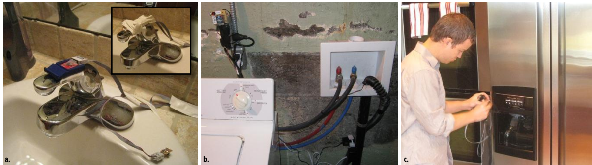
Figure 8.3: (a) Accelerometers were used on single handle faucets to track flow and temperature position; (b) A modified Kill-a-Watt tracks the laundry machine’s energy use to indirectly monitor water consumption—a thermistor was placed in the drain pipe to discriminate temperature settings. (c) In H1, we used a reed switch configuration to track refrigerator dispenser water usage.
